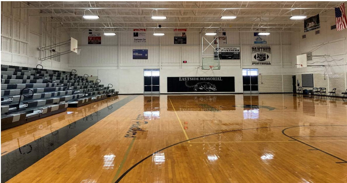
The main gym is too small to support bleachers on either side of the playing area and lacks dedicated restrooms.
