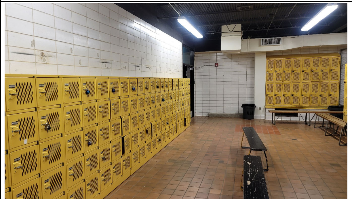
Boys' and girls' locker room is dated and in poor condition
