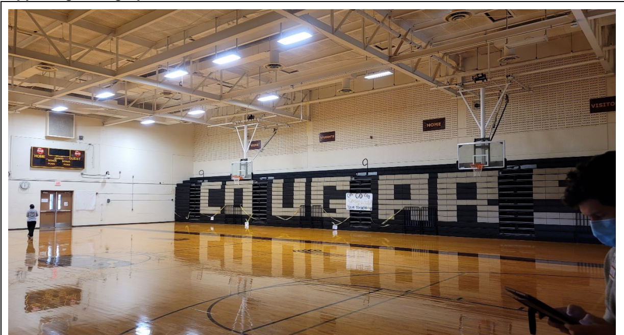
Main gym is in average condition despite being original to the school.
