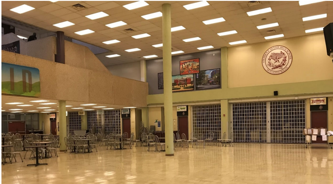
Cafeteria is undersized for campus capacity and cannot hold events such as banquets for student groups. Fluorescent lighting throughout the school is dated and not controllable.
