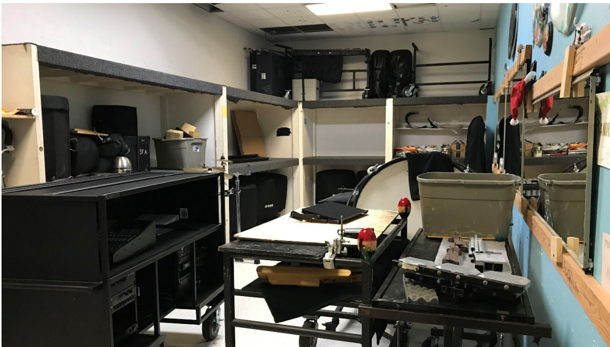
Throughout the school there is a shortage of storage. Many storage areas are cramped and difficult to navigate.
