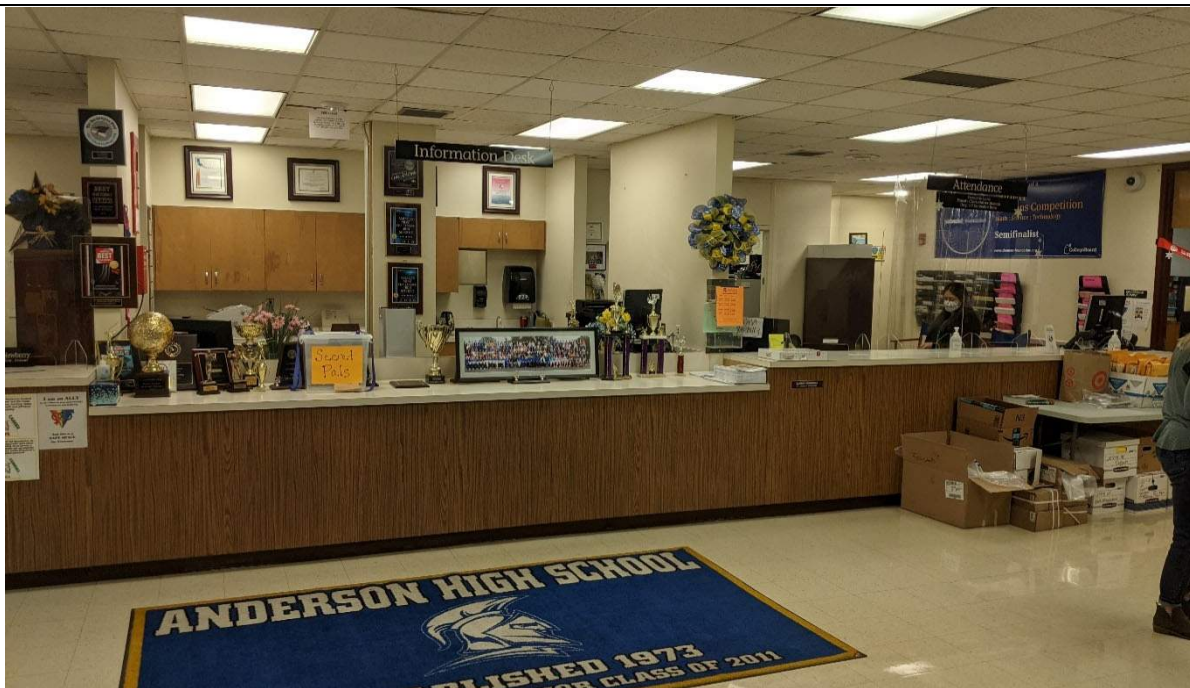
Administration: Large reception, but finishes are dated and does not feel welcoming.
