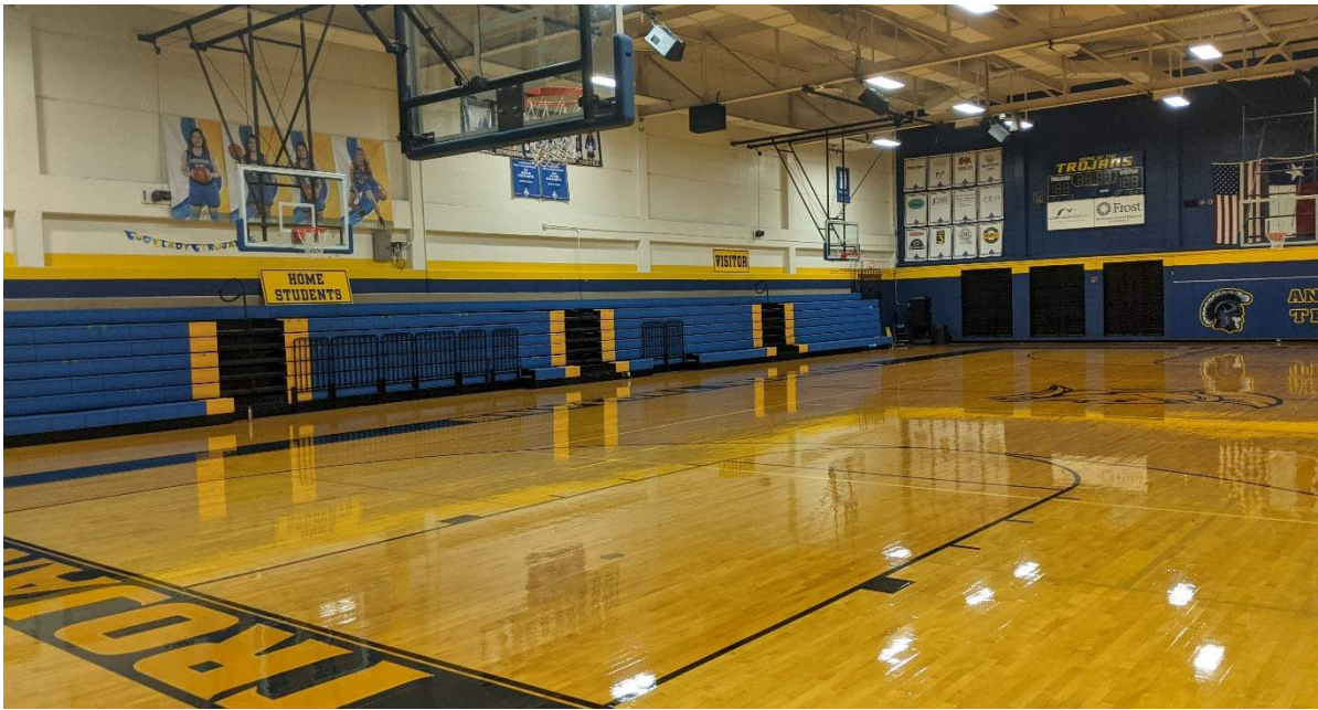
Athletics and Wellness: Gym does not meet current Ed Spec but is in good condition. It is significantly smaller at 10,100 SF than the 16,400 SF per Ed Spec.
