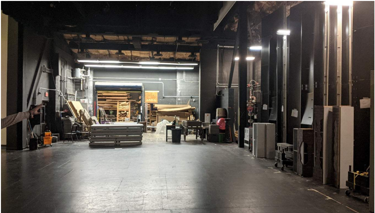
Visual and Performing Arts: Theater stage with attached scene shop. The theater has recently undergone electrical upgrades via private donation. The stage and wing space are undersized per Ed Spec. It was also noted by Fine Arts Director that the proscenium is not wide enough for a modern theatrical production.
